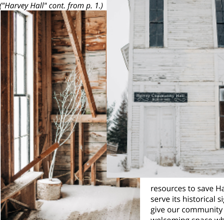
The snow on the floor highlights the need to fix the leaky roof. Photos on page 3 by Madeline Taylor.
